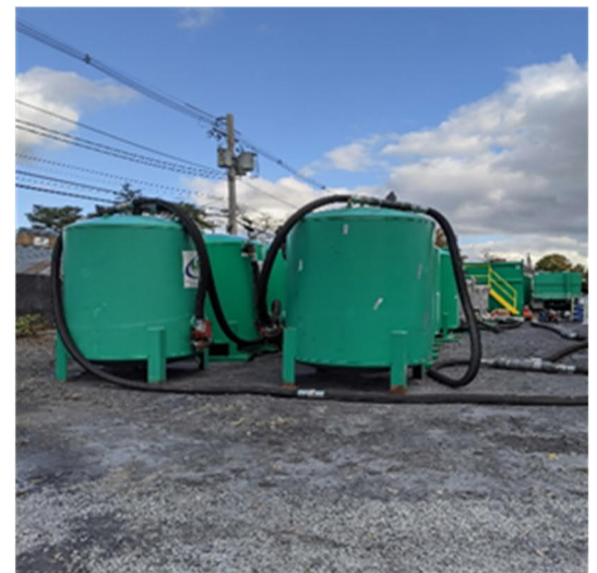
Water Treatment System
